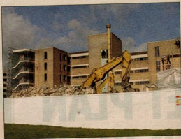
COMING DOWN Davis House being demolished in February as one of the sites for the regeneration project
