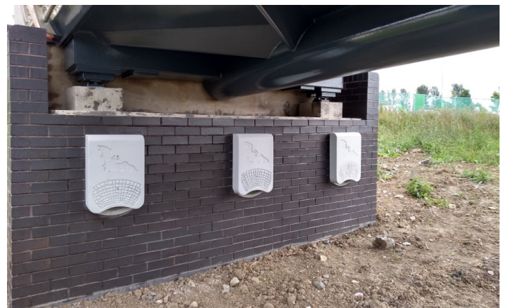
Bat boxes installed under the bridge at the Hall & Woodhouse. Credit: Chris Barry
